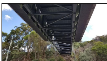
Figure 13. Exterior view of the underside of the pedestrian footbridge. Taken from the south side of Wentworth Avenue, facing north-east.
